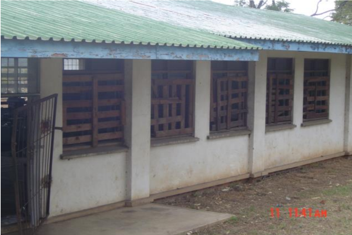
Fig. 5 Showing how some school workshops have dilapidated over the years even looking from outside
